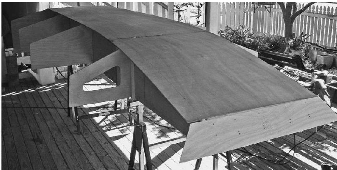
The bottom, previously butt-jointed, is attached to the framework. Note the neatly countersunk holes for the fasteners.
