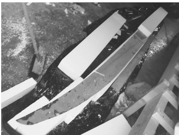
FIGURE 8-22. Foam blocks being glued to a plywood shear web. (Photo courtesy Marc Termonia)
