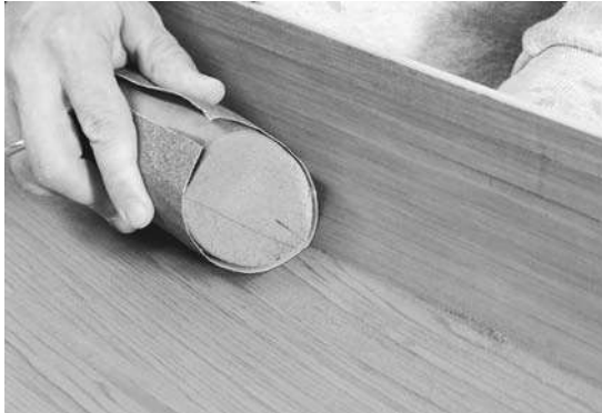
Figure 7-13. A fairing sander does not work well on interior surfaces, but after scraping and planing, you can get a quite fair surface by wrapping sandpaper around a chunk of soft foam or a shaped wooden sanding block with some foam cushion on it.
