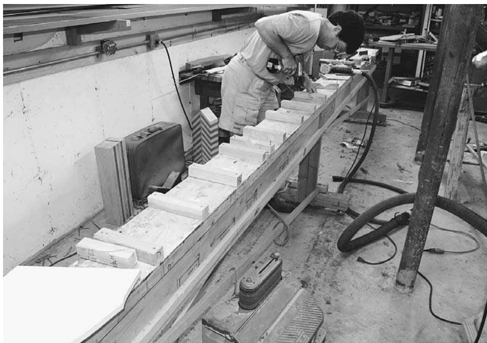
Figure 5-20. Forms are attached to an external strongback with wooden cleats. Mark the strongback with the appropriate spacing with a centerline marked in place. Screw the cleats in place next to the spacing marks.
