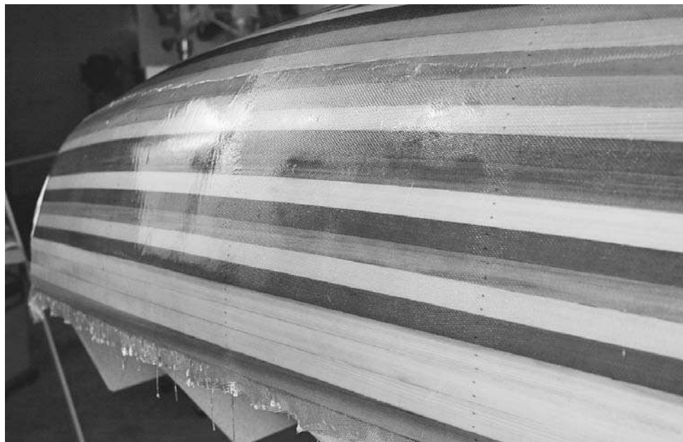
Figure 9-27. The fill coat fills up the fabric texture (right) to create a smooth finish (left). There are several methods for doing this: some are quicker but open you up to making a mess; others are more controlled but time consuming. I brush on the epoxy using the same crisscross technique I use to apply varnish.
