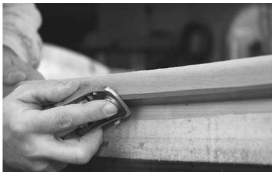
Figure 11-35. The edges of the outwale all start out with sharp corners. First plane down the exposed strip along the top edge so it is even with the outwale. Then use a round-over router bit to give the top edges a radius. The bottom is not at 90 degrees to the outer edge, so a standard round-over bit doesn't do the job. Instead, round it over by hand with a block plane. First create a wide chamfer, then knock the corners off the chamfer and sand it all smooth.
