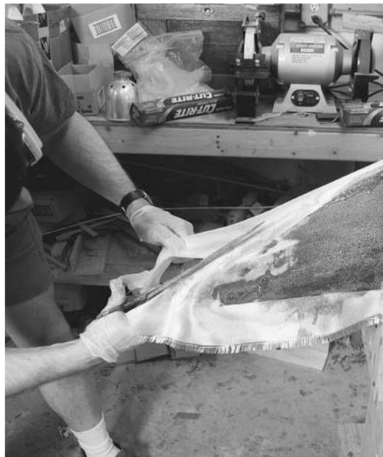
Figure 9-17. Most wrinkles need to be moved toward the ends of the boat. Depending on the shape of stem, you may need to trim the glass at the ends. While it is possible to wrap the trimmed glass around either side, I find it easier to let it come off straight and then trim it off later.
