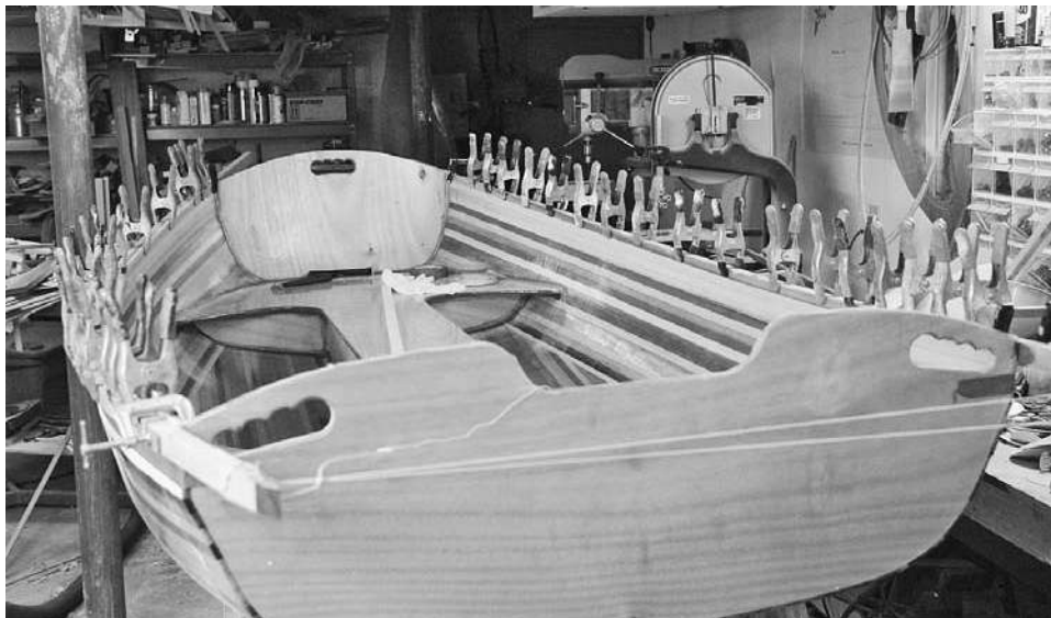
Figure 11-34. I installed an outwale only. Having no inwale makes it easier to drain the boat. Glue the outwales to the sides of the boat by applying a layer of epoxy thickened with colloidal silica. Spread the mayonnaise-consistency glop on both the boat and the gunwale stock. Protect the side of the boat below the gunwale with masking tape so drips won't make a mess. Install the outwale just below the top edge of the strips.
