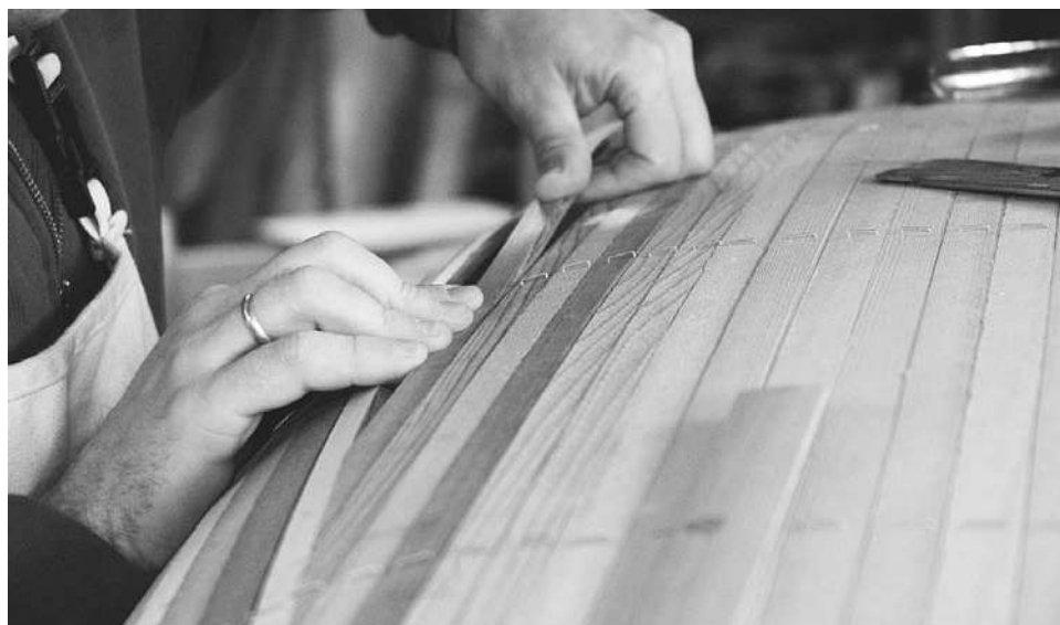
Figure 6-32. With cove-and-bead strips where you are fitting both ends of a new strip, the strip ends up being longer than the visible gap because the strip extends down into the cove of the prior strip. Thus you cannot just drop the fitted strip into place; you must snake it in. It can also be very difficult to remove a strip after dry-fitting it. Instead you will want to rely on accurately making the alignment mark described in Figure 6-27. When you have successfully dry-fitted each end separately and the alignment mark lines up perfectly, add glue to the strip, insert it at one end, then bow it up in the middle to shorten it enough that you can slide the second end in place. The strip should then snap into place.
