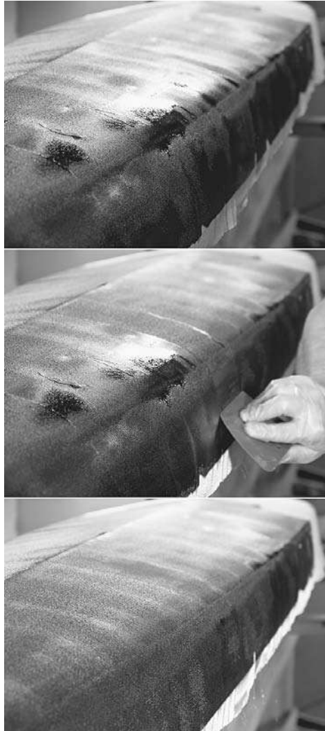
Figure 9-19. After wetting out the glass there are bound to be areas with excess resin as well as some with too little. Starting at the center-line, hold the squeegee at about a 45-degree angle. Pull the squeegee toward the edge, maintaining approximately the same angle as you roll down the side. Clean the epoxy off the squeegee by sliding the edge through a slot in a paper cup.
