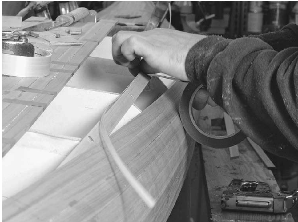
Figure 13-30. The deck has a feature line, or crease, near the cockpit. I wanted the strips to look like they go straight across this crease, but I also wanted to put a light-colored accent strip at the crease. I installed a temporary strip below the feature line to support the ends of the strips above the feature line. I also cut a very thin strip of maple. Here I am temporarily taping this thin strip of wood to the temporary support strip. This will create a light-colored strip in the finished boat. As I fill in the strips above the feature line, I will glue their ends to this maple piece, removing the tape as it gets in the way. After I have finished filling in above the feature line I will remove the temporary support strip and fill in below. The thin maple strip will remain in place.
