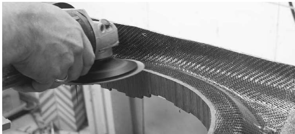
Figure 13-52. When you turn over the deck you can trim off the bottom ends of the coaming riser strips. First clean out any hot-melt glue squeeze-out. The glue will quickly gum up any sandpaper or rasp. I use a high-speed right-angle grinder to bring the strips down even with the deck interior. A 36-grit disk makes quick work of the task even if it does send dust everywhere. You need to be careful, as it will grind through anything without a second thought. The disk may also be handheld to round over the edge after it has been trimmed.
