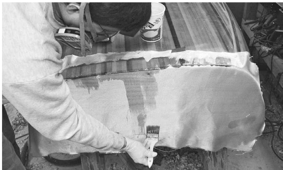
Figure 11-23. The glass on the transom extends a couple of inches onto the strips. Note the use of blue tape to make a clean edge. The end grain of the strips absorbs a lot of resin, so either keep adding more or do a seal coat before starting the glass coat.
