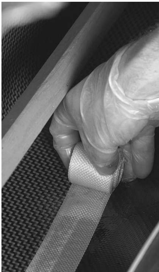
Figure 13-69. Bonding the deck-hull seam is no fun, but it is over quickly, and it is really the best, strongest, lightest solution. As described in Chapter 9, you must run a length of prewoven tape down the inside seam. Here I am using a 1½-inch wide Kevlar tape. I'll roll it by hand as far down the seam as I can reach, then break out the brush-on-a-stick.
