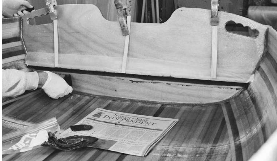
Figure 11-32. The intersection of the backseat and back transom will need some reinforcement. Normally I would create a fillet underneath, but the only access to this area will be a small hole in the seat support. Therefore, I opted to make a fillet before installing the seat. You could glue and screw a cleat of wood into this position, but I like the rot resistance of a fillet in this location. A solid piece of wood as a cleat could be covered with fiberglass and epoxy to protect against rot, but this method is quicker.
