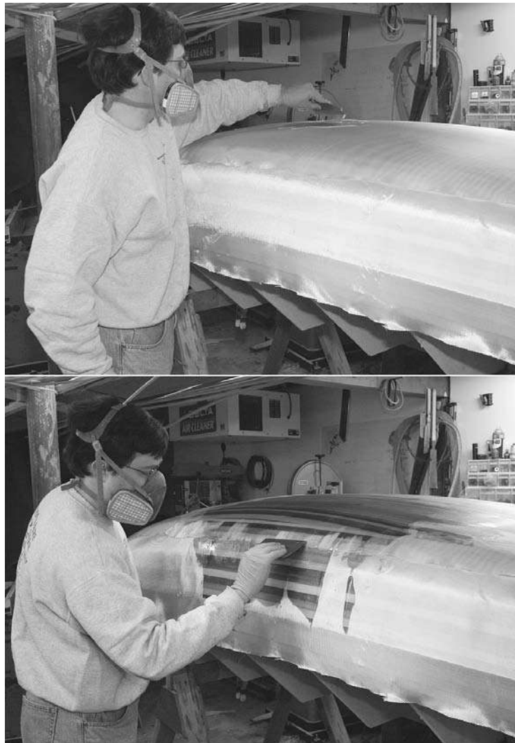
Figure 11-19. Cover the boat with 6-ounce fiberglass. The two layers on the bottom will soak up quite a bit of resin. Pour a puddle of epoxy on the bottom and spread it around with a squeegee. Work from the middle, down the sides, and then out toward the ends.
